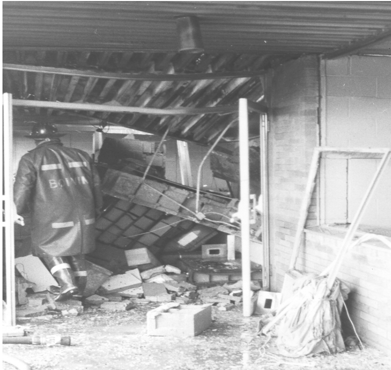
East Wall of Education Wing After Explosion.
